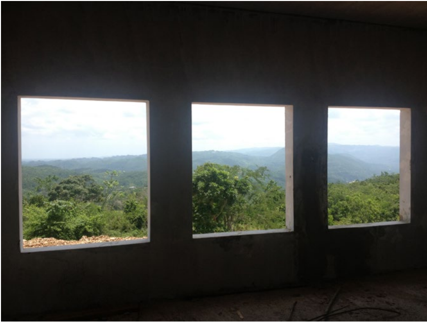
Figure 13.5 Inside the building site: large rear windows overlooking hill precipices are focal points in houses like these. Photograph by Davinia Gregory, July 2013.
