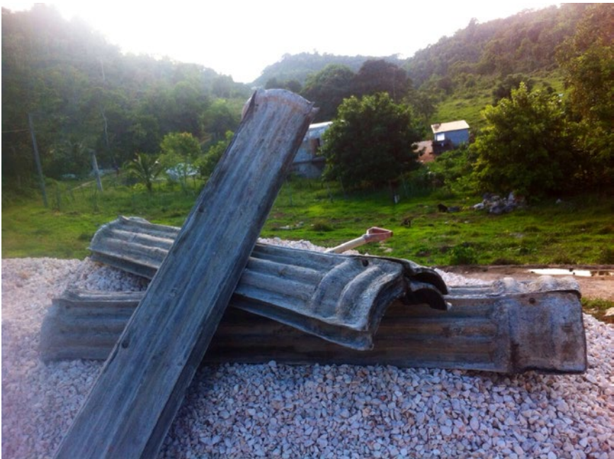
Figure 13.3 Metal column molds on a building site. Photograph by Marie Hayden, November 2014.
